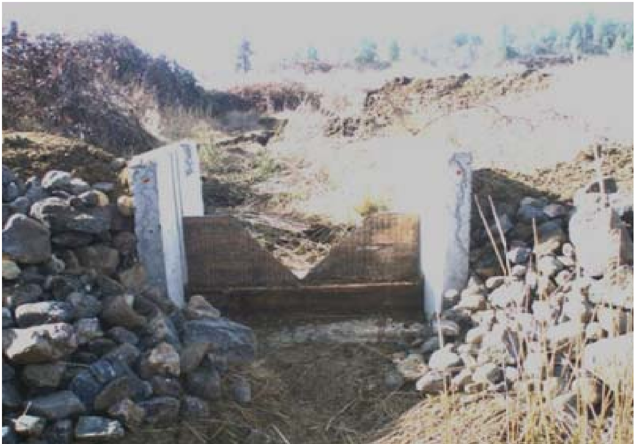
Figure 3. Precast box & V-notch weir with rip-rap.
